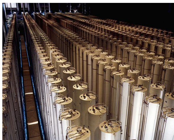
Figure 3. Picture of centrifuge plant in practice.
